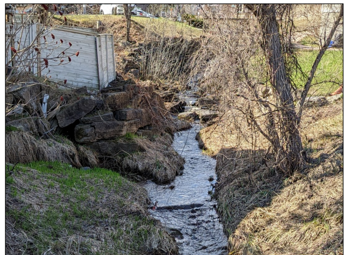
An example of the use of armourstone on a headwater drainage feature on Robertson Road
