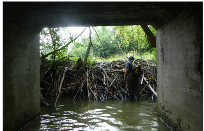
An active beaver dam blocking the culvert under the railway east of Moodie Drive
