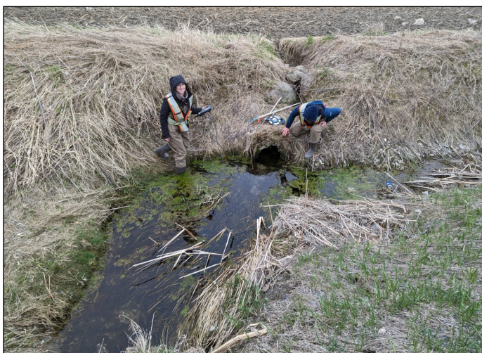
RVCA staff assessing a headwater drainage feature in the Mud Creek catchment.
