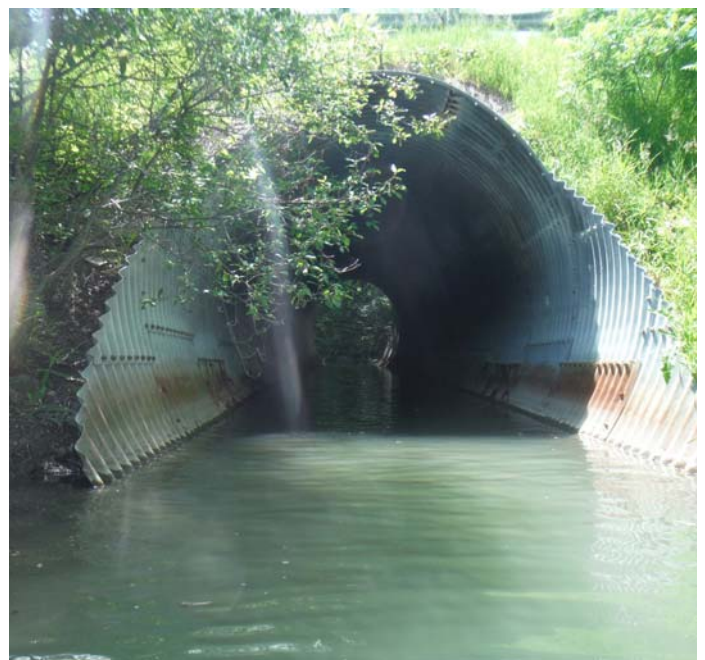
A highly altered section of Black Rapids Creek where it crosses Merivale Road.
