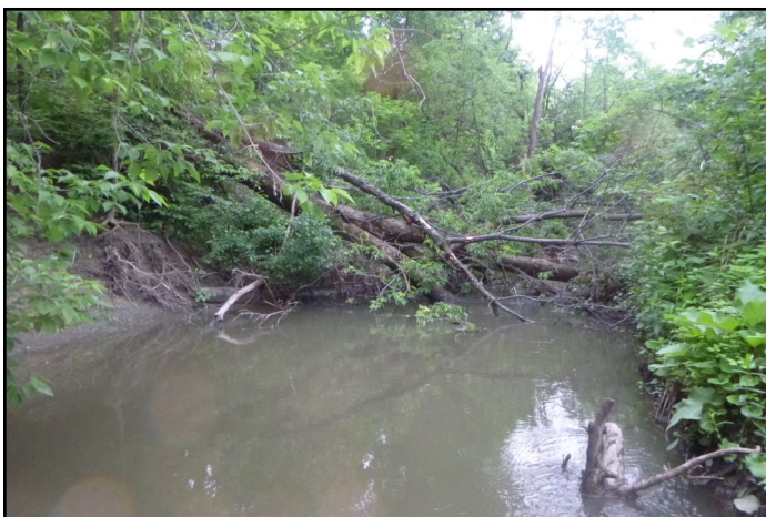
Bank erosion exposing tree roots, creating instability for trees along the left bank of Sawmill Creek.
