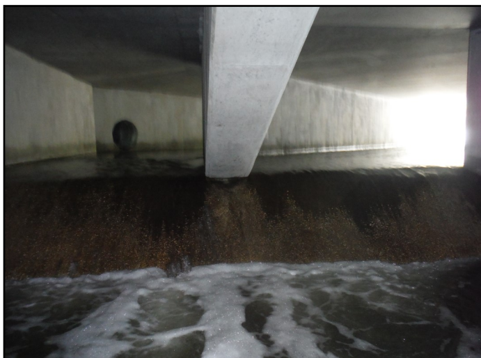
Perched culverts can result in fish passage obstructions which can reduce species diversity along a watercourse.
