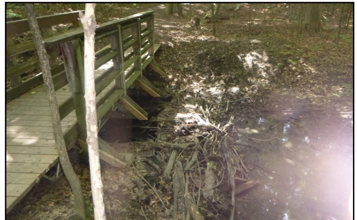
Debris jams in the upper reaches of Barrhaven Creek, create seasonal migratory obstructions.
