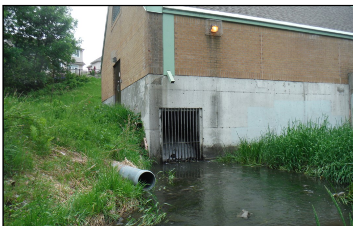
Building structure at the stormwater management facility on Barrhaven Creek is a permanent migratory obstruction.
