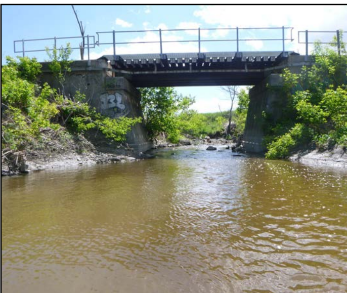
Section along Ramsay Creek with forest, scrubland, meadow and railway infrastructure land uses west of Ramsayville Road
