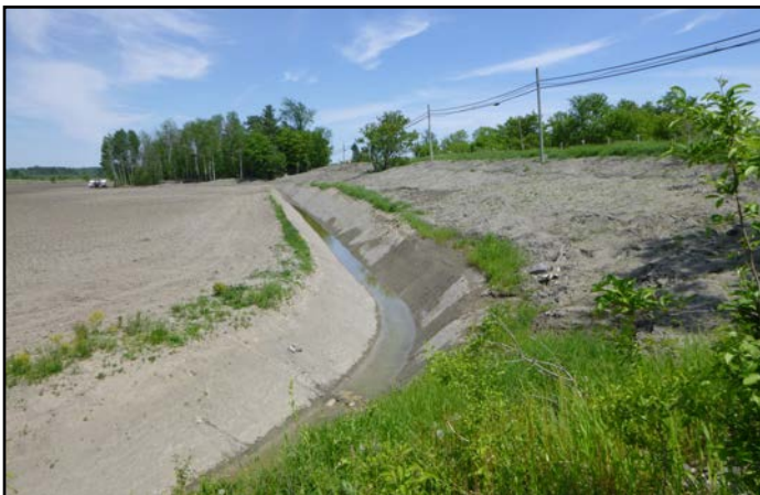
Branch of Ramsay Creek that would benefit from channel enhancement north of Russel Road
