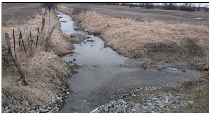
Substantial sediment deposition observed in a headwater drainage feature on Anderson Road
