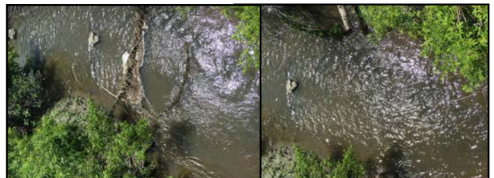
Before (left) and after (right) the removal of abandoned communications lines on Ramsay Creek near Ramsayville Rd
