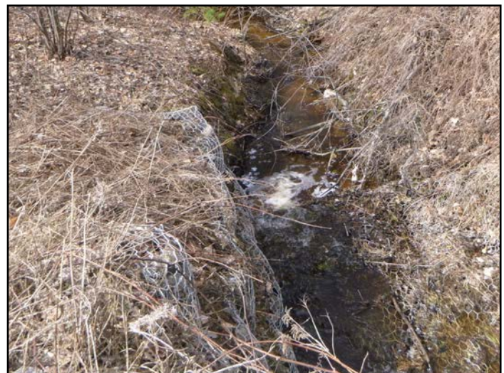
An example of the use of gabion baskets on a headwater drainage feature on Anderson Road
