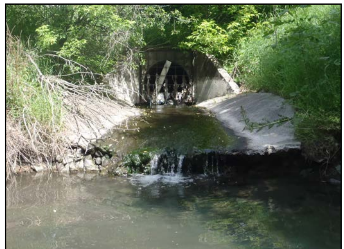
Stormwater outlet partially blocked with garbage and debris; out-letting into Nepean Creek
