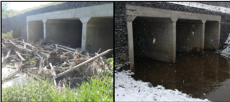
Debris Jam obstructing the entire stream at St. Joseph Boulevard bridge, brought to our attention by Adopt-A-Stream volunteers in Greens Creek (left). This City of Ottawa removed this debris in late fall of 2016 (right).
