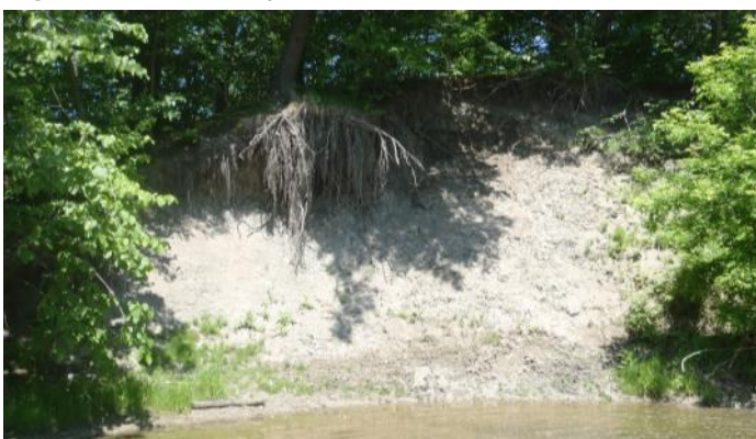
Stream bank erosion along Mosquito Creek
