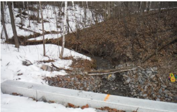
HDF with no vegetation due to rip rap in the channel
