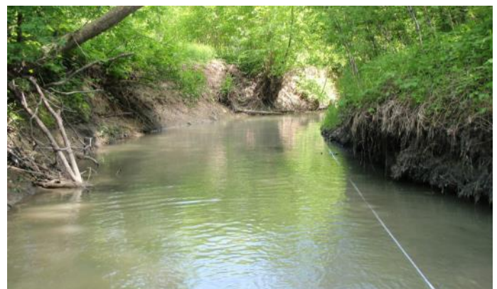
Bank undercutting on the right bank and erosion on the left bank of Bilberry Creek
