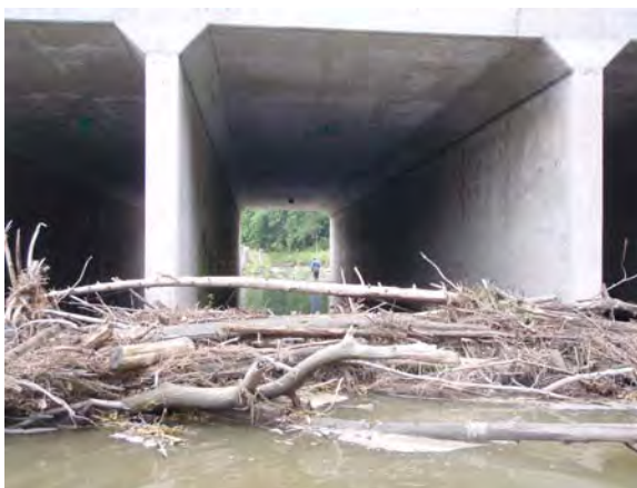
Triple box culvert at St. Joseph causing log jams
