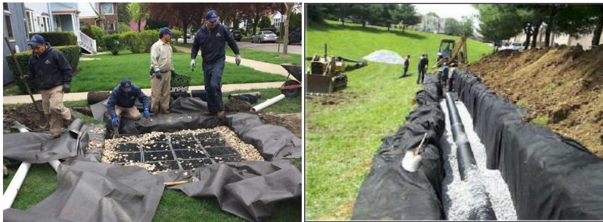
Figure 4: Left: Residential soakaway pit (City of Ottawa, 2022). Right: Infiltration trench example from Cahill Associates (CVC & TRCA, 2010)
