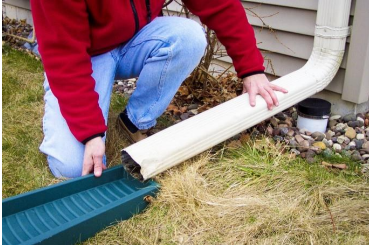
Figure 6: Downspout disconnection, extender, and splash pad (Alliance for the Bay, 2022).
