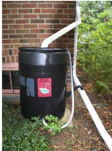
Figure 5: Typical residential rain barrel set up (CVC & TRCA, 2010)
