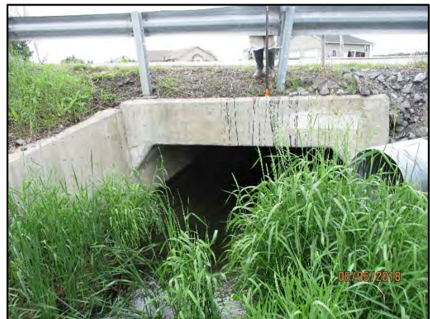
Roger Stevens Drive and 3 rd Line Rd (Downstream)
